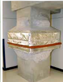
Fire blankets were used in Channing House.
